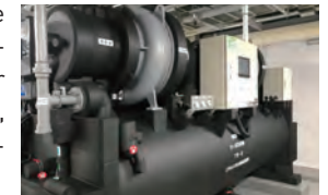
Water chiller freezer at the Urawa Factory
